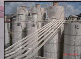
Inlet piping of the silos
