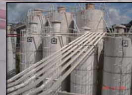
Inlet piping of the silos
